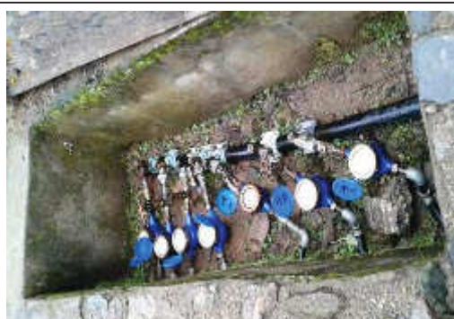
4. Meter Installation Point for 24 Hour Water Supply to Main Offices
