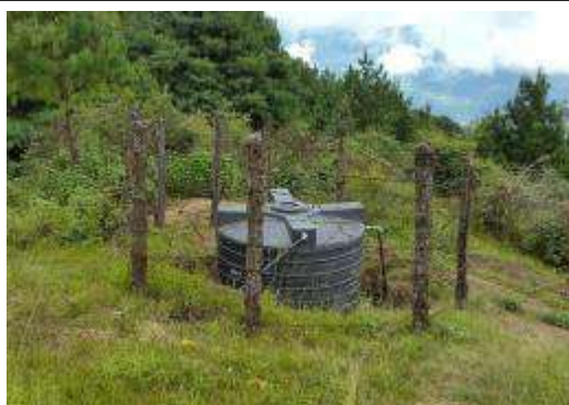
13. Existing WS Scheme near Tower
