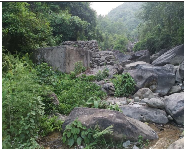
Existing Collection Chamber, Betai Khola ward no.2
