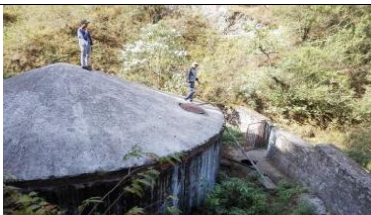
Existing RVT of Khalanga Bazar System at ward no. 4
