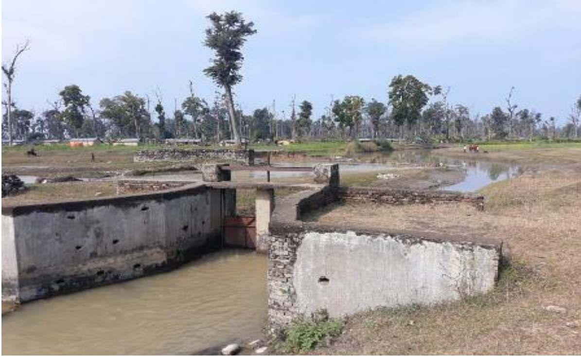
Division Section of North Gyani kulo and South Gyani kulo in the end point of Jamara Canal
