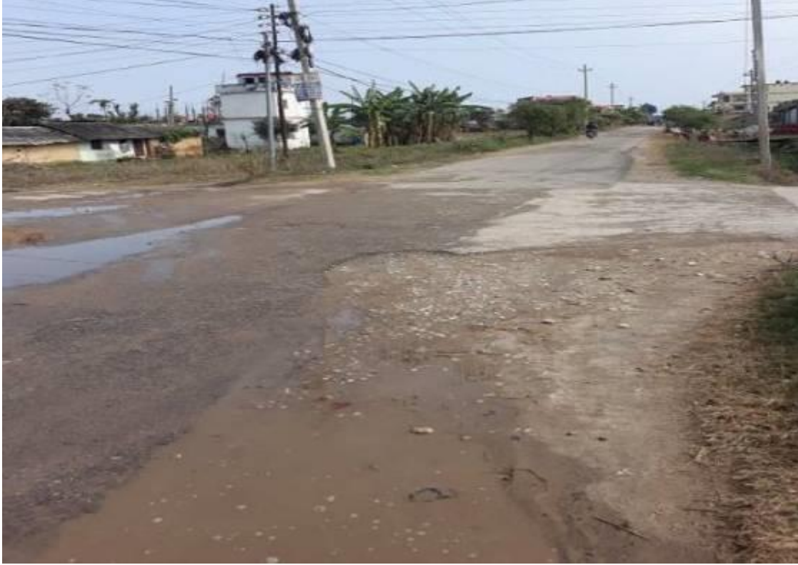
Proposed public/government Road ROW for Drain construction at Shaktinagar area, Tikapur municipality ward no.1
