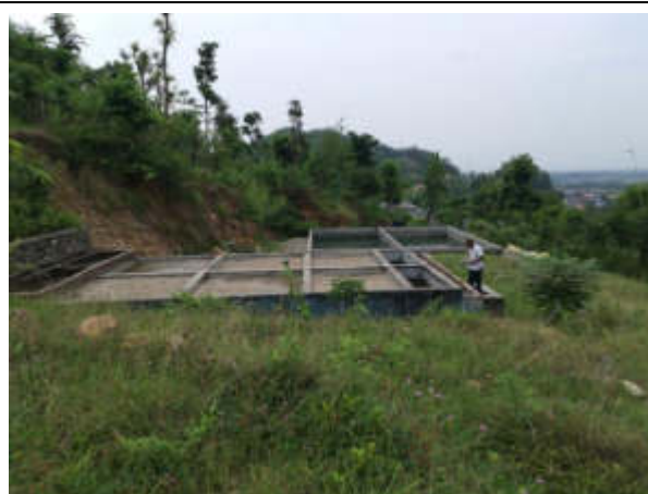
6. Existing Water Treatment Plant, Pathar Khola (Shivalaya)
