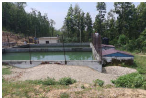
8. Existing Water Treatment Plant, RVT-1 site(Dihi Danda)
