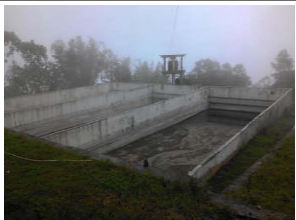
4. Existing WTP at Charkhade
