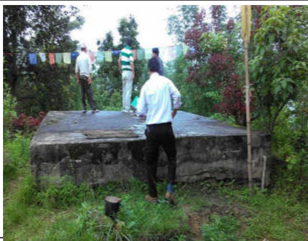
5. Existing Water Tank at Gumba Danda that needs rehabilitation
