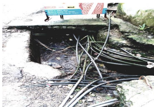
8. Existing condition of distribution pipelines
