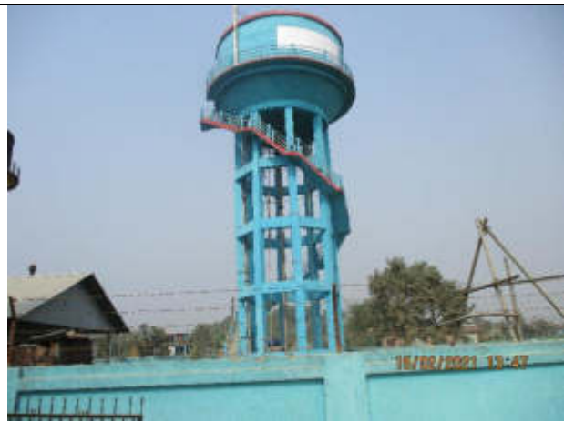
Photo no. 2: Existing OHT, (225 Cum) in WUSC compound at Pani tankey Ramdhuni Municipality ward no 3
