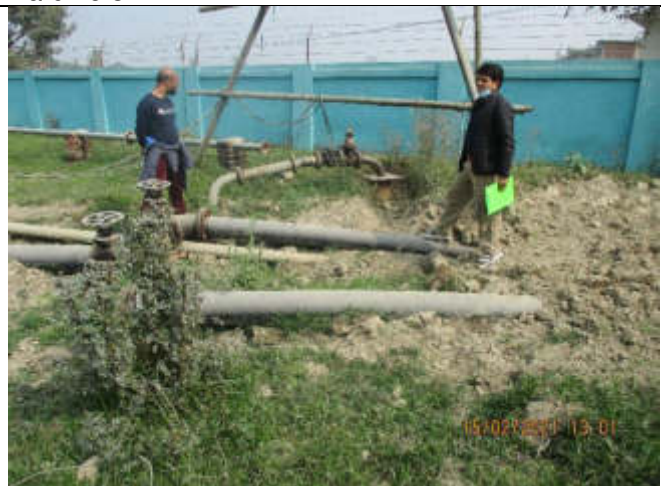
Photo no. 4: Existing WUSC compound and proposed two deep boring sites at Pani tankey tole ward no 3
