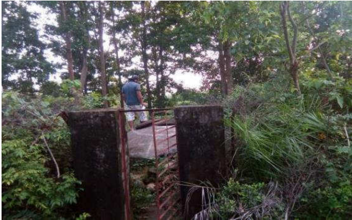
Photo 5: Reservoir of Existing Singhe System
